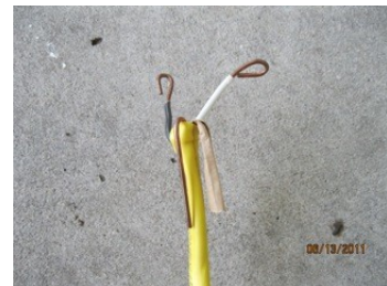
Illustration 13: Stripped electrical wire with looped ends. Note that the ground wire is folded out of the way.
