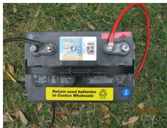
Illustration 17: Note that the POSITIVE (+) BATTERY POST is clearly marked with RED TAPE.
