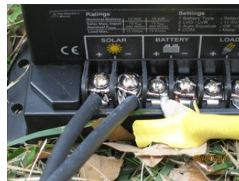
Illustration 8: Solar panel connection is on the left. The battery post connections are also shown.
