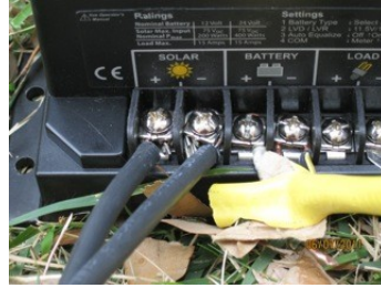
Illustration 10: Solar panel connection is on the left. The battery post connections are also shown.
