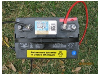
Illustration 15: Note that the POSITIVE (+) BATTERY POST is clearly marked with RED TAPE.
