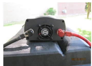
Illustration 20: Looped-end battery cables connected from the battery to the inverter.
