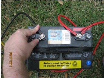
Illustration 18: Note: The PAIRED LOOP END BATTERY CABLES from the SunSaver AND the INVERTER are connected onto the same BATTERY POSTS.
