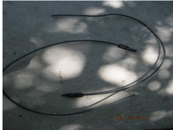
Illustration 4: Solar panel connectors with open wire ends.
