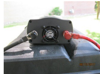
Illustration 18: Looped-end battery cables connected from the battery to the inverter.
