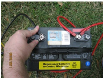
Illustration 16: Note: The PAIRED LOOP END BATTERY CABLES from the SunSaver AND the INVERTER are connected onto the same BATTERY POSTS.
