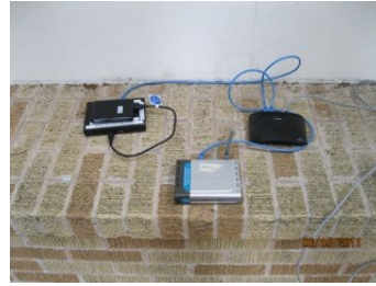
Illustration 5: Left: Genesi SmartTop with the 500 Gigabyte external hard drive on top. Center: D-Link AirPlus G Router. Right: D-Link 5 Port Ethernet Switch.
