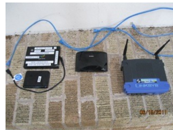
Illustration 12: Components without the Rocket M5 in view. Note that the 5 Port Ethernet Hub is not in use.
